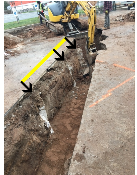
Trench to electrical room had to go through previous house basement foundations. They had to be jackhammered out.
